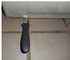
no sealant around grease trap
